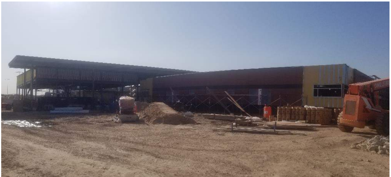
Segments F & H (8 th Grade Wing & Kitchen) – Brick veneer and exterior framing
